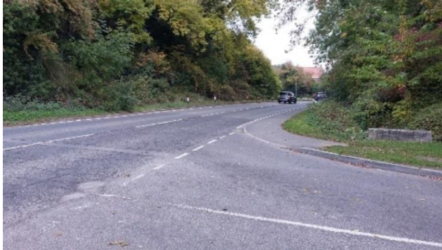
Figure 3: Photograph from junction of Park Lane/Nottingham Road with trees/vegetation obstructing visibility splays
